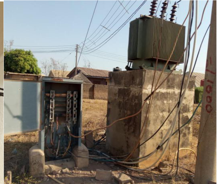
Distribution Lines @ JED, Gboko
