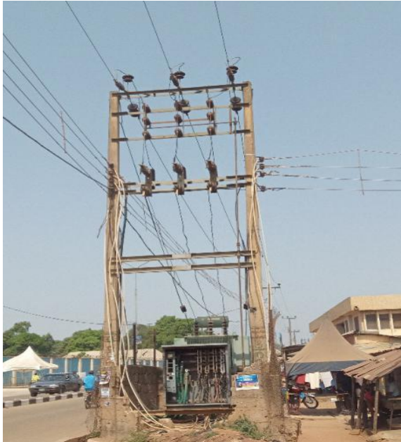
Step-down Transformer @ Gboko, JED
