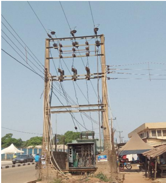
Step-down Transformer @ Gboko, JED
