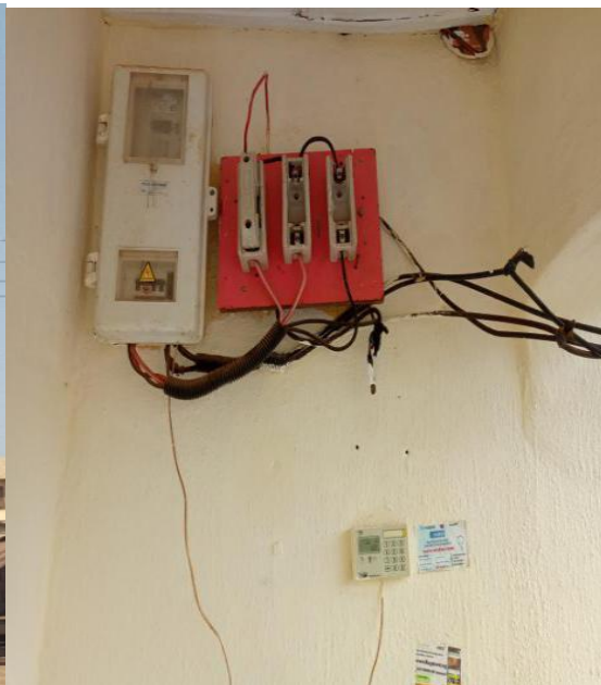
3-phase Residential Meter @ Karu LGA,
